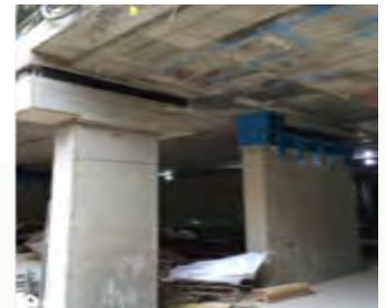
Fig 9.2 Vertical Support Bearings
