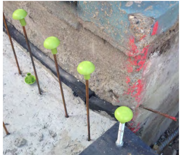
Fig 10.7 50 mm Thick Farrat ISOFOAM IS12 This was used to laterally separate the isolated building from any surrounding, non-isolated structures.
