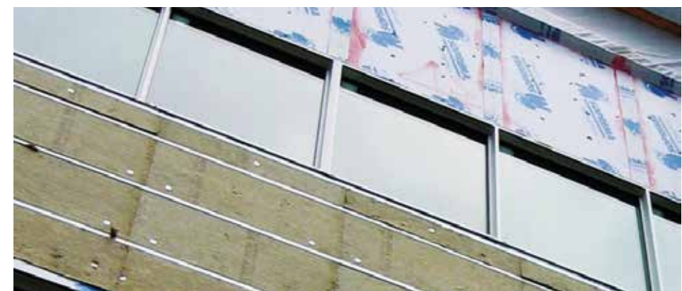
Exterior insulation installed in-between steel z girt cladding support attachment resulting in exterior insulation that is not continuous and does not meet energy codes (Source: Roxul, Inc.)
